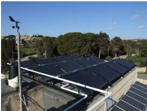
Figure 8: Vacuum tube solar collectors on the left and PV panels on the right.
