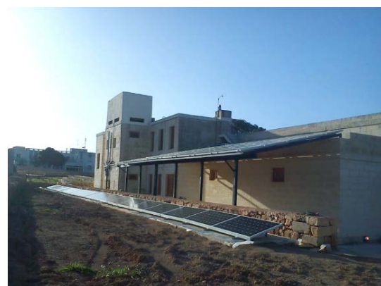
Figure 3: Photograph showing the PV arrays
