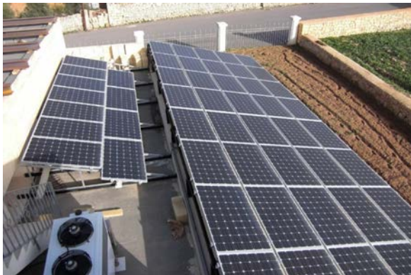
Figure 6: The PV arrays on the roof of the building and on the canopy.
