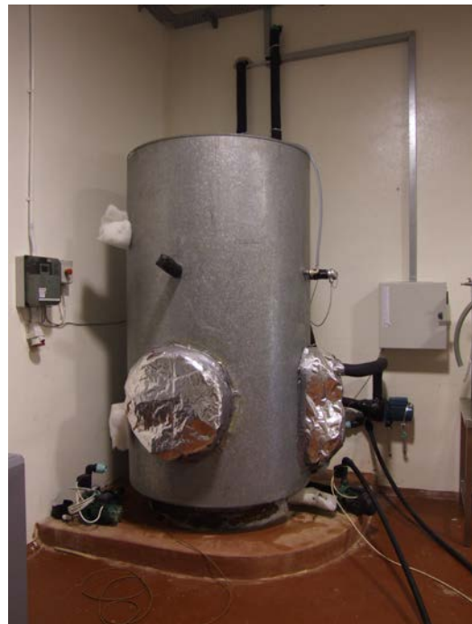
Figure 12: The cold water storage tank, with the DAQ box on the left, a power meter on the right.
