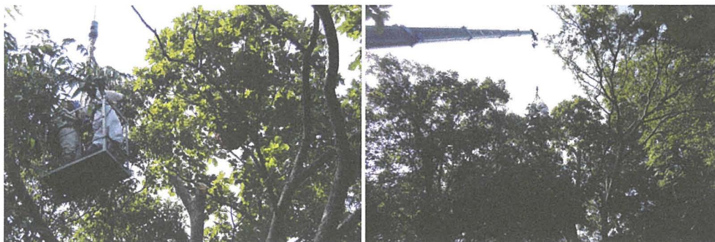
Figure 68. Crane lifts two professionals on a platform high up into the canopy to remove an Asian hornet colony. Photographs by J. Takahashi.
