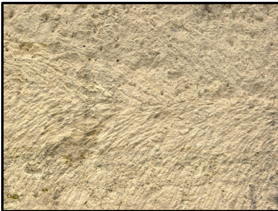
Figure 57. The limestone texture with distinctive toolmarks chosen to texturize the reconstructed mesh of the hypogeum (Texture Library 2022).
