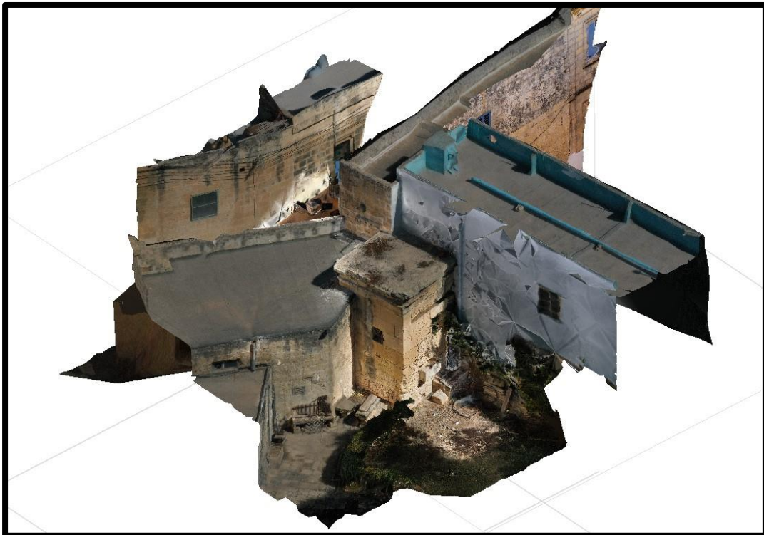
Figure 105. Screenshot from Agisoft Metashape showing the built textured mesh of the reality-based 3D model (photo by the author).
