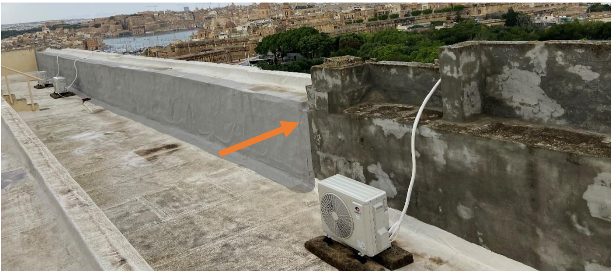
Figure 66. Arrow indicating the limit of the footprint allowed in the past whilst using the roof.
