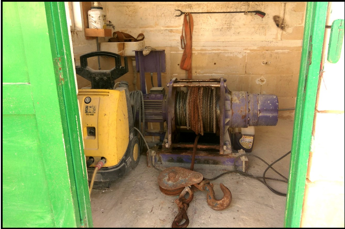
Picture 7: The mechanical winch inside the room (Source: my own)
