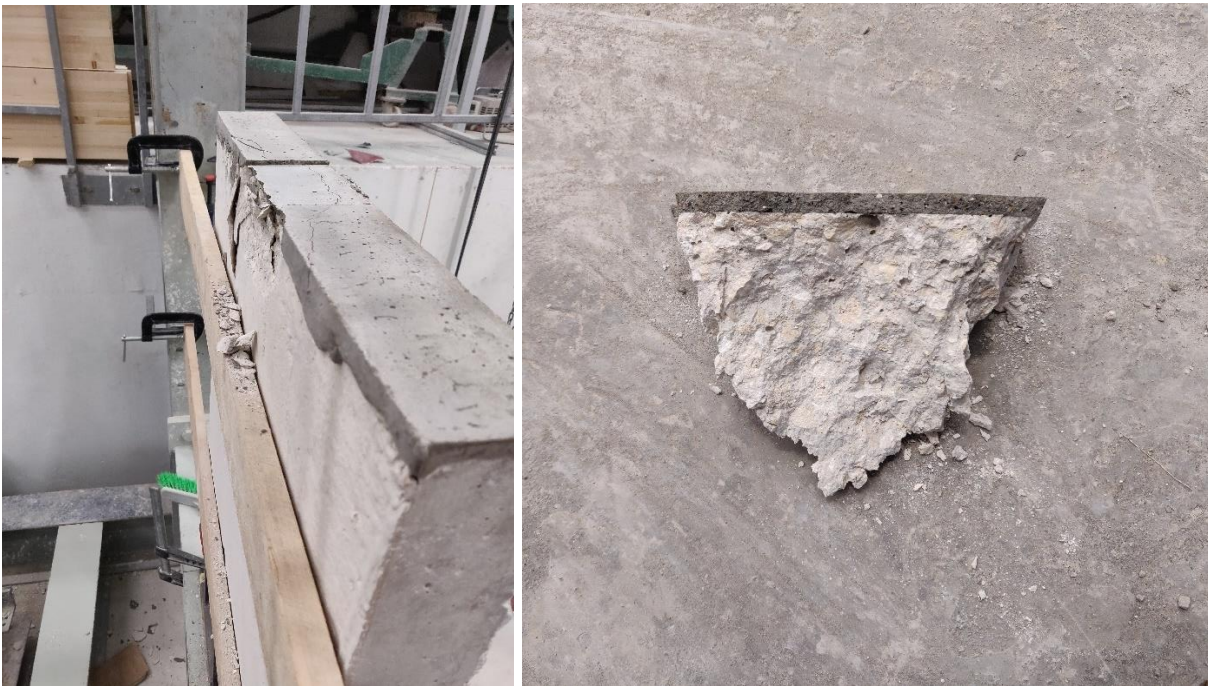
Figure F.43 – Concentrated load failure mode through the grout layer, forming a cone/wedge
