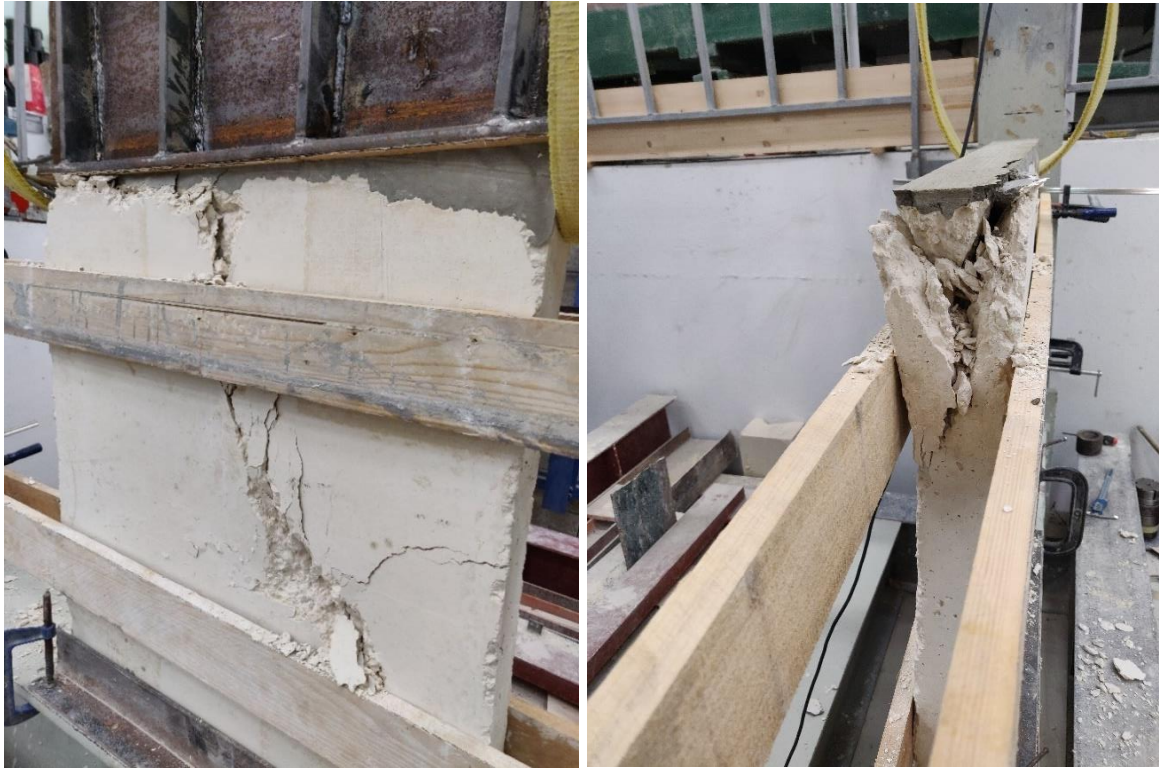
Figure 4.9 – Left; failure mode back elevation; right, diagonal cracking through the top surface
