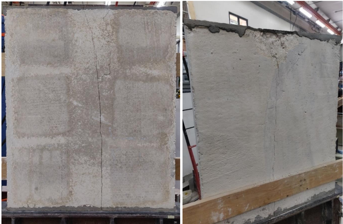
Figure 4.53 – Left , failure mode front elevation; right , failure mode back elevation
