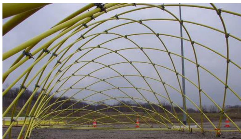
Figure 2.27: A large scale prototype of the grid shell developed by Douthe, Baverel and Caron
