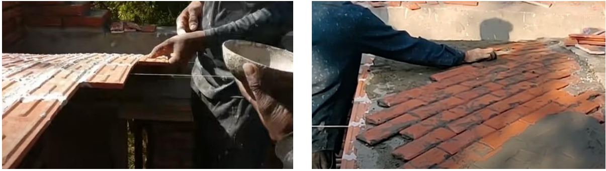
Figure 3.19: Left: First layer of the Catalan vault using rapid setting mortar; Right: Application of the second layer at a 45 degrees angle
