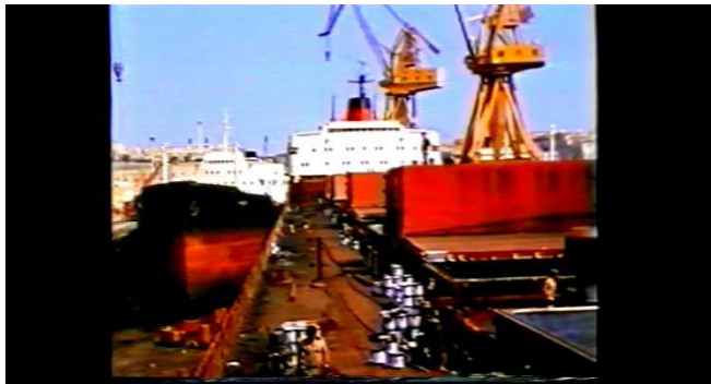
Fig. 107: Scene of work in progress at the drydock in the Grand Harbour
