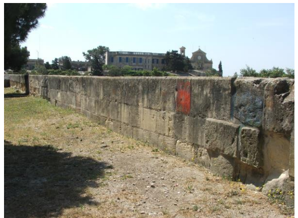
Pollution encrusted recent alterations on parapet.
