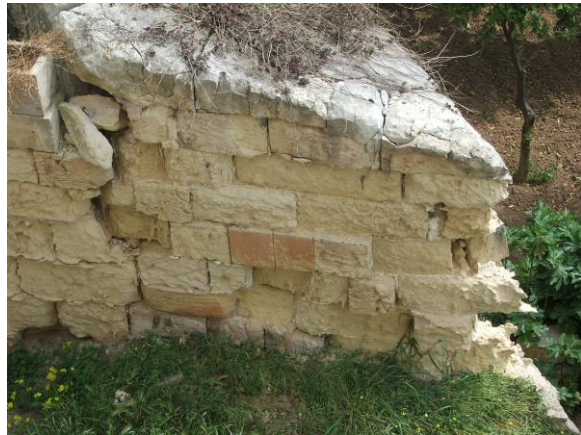
Fissure, broken stone and mass deterioration.
