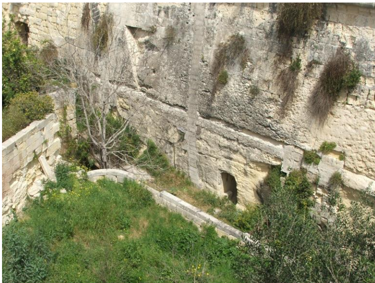
Trunking, black crust, biological and plant growth, excavated shelters and concrete on the rock-hewn face.
