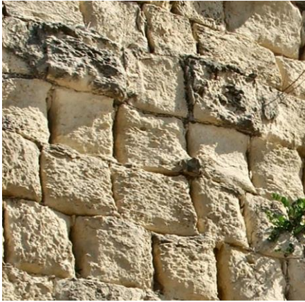
Fig. 10. Crumbled masonry on left scarp.
