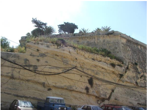
Badly eroded rock hewn face remaining stones.
