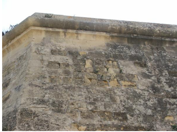
Fungal growth, black crust and eroded stone.
