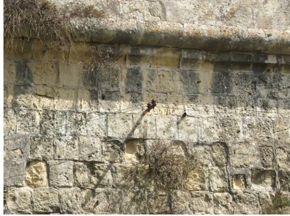
Fig. 49: Algae, black crust, growth and accretions along the right scarp.
