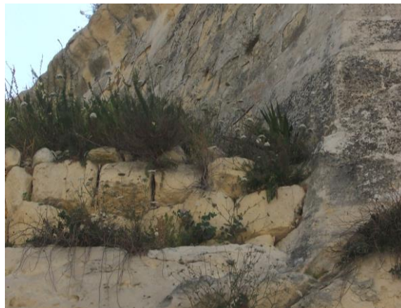
Badly eroded stones and overgrown with plants.
