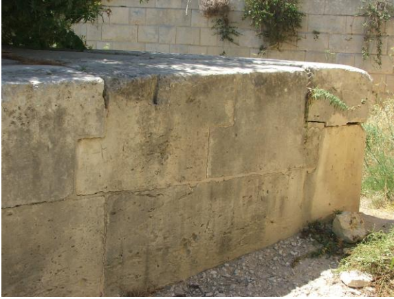
Dislodged quoins on the face of an embrasure.
