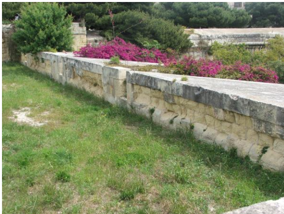
Badly eroded parapet and missing banquette.
