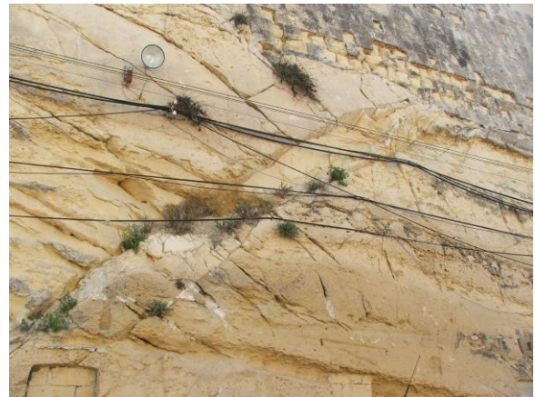
Fig. 15: Faster deteriorating weaker strata and accretions on the rock-hewn lower face.
