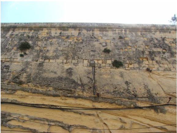
Fig. 14: Rich deposits of encrustation on the right face, which has fallen where the stone or rock is powdering.
