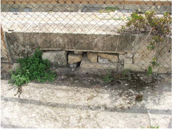
Fig. 15: Concrete and other accretions along the parapet and inside the expense magazine.
