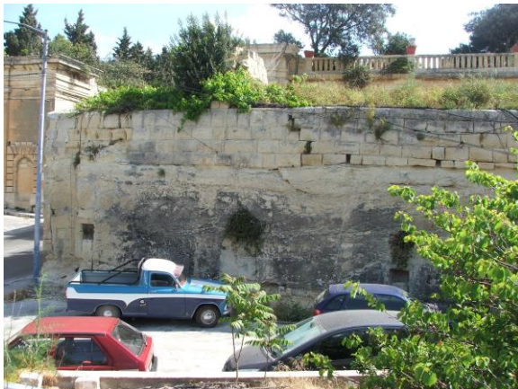
Black crust, crumbling masonry and plants.
