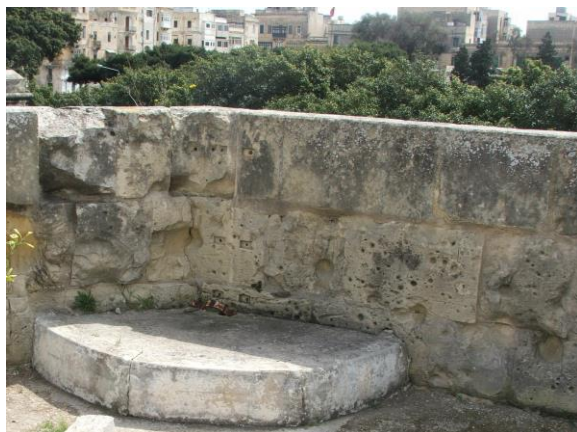
Shrapnel damage on orillion's parapet.
