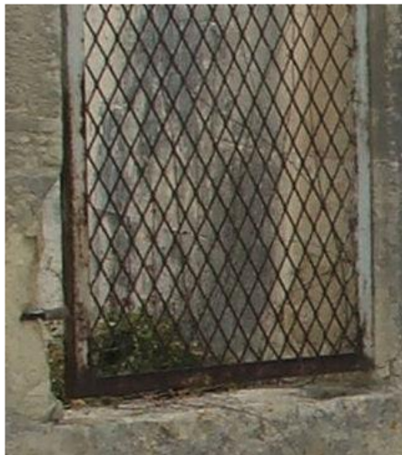
Fig. 22: broken and crumbling stone and cheeks caused by rusted safety mesh.
