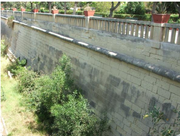
Deterioration on the modern 'curtain' face.
