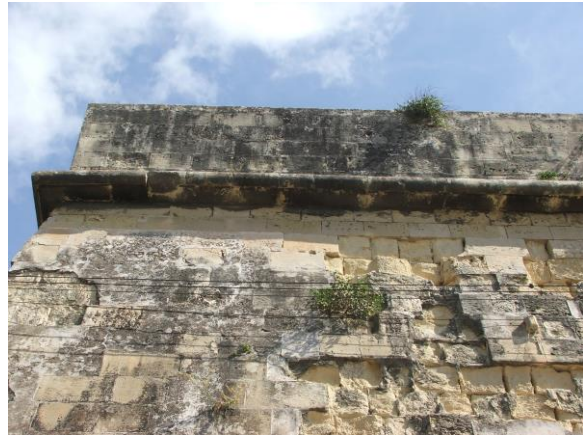
Fig. 11: Delamination, powdering, crust and growth.
