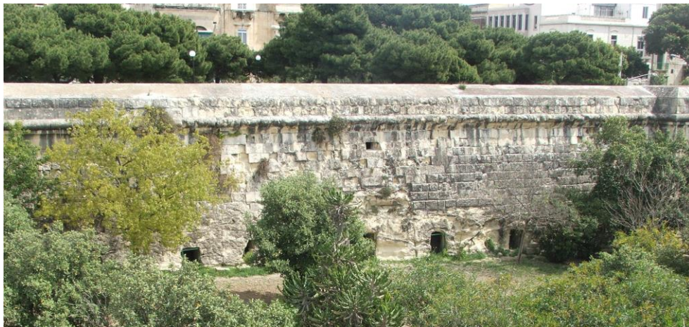
The various interventions and types of deterioration on St. Anne's Curtain.
