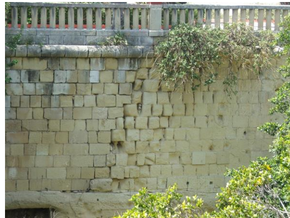
Post war restoration and bulging masonry.
