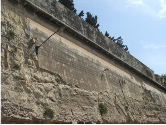
Fig. 12: A replaced section of the left scarp and parapet showing algae growth and encrustation. Or was this section damaged during WW2?
