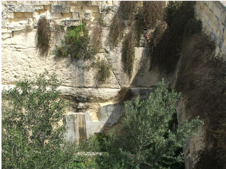
A little of everything; Alveolar erosion, powdering stone and rock face, broken or leaking water drains, concrete rendering and intense plant growth.
