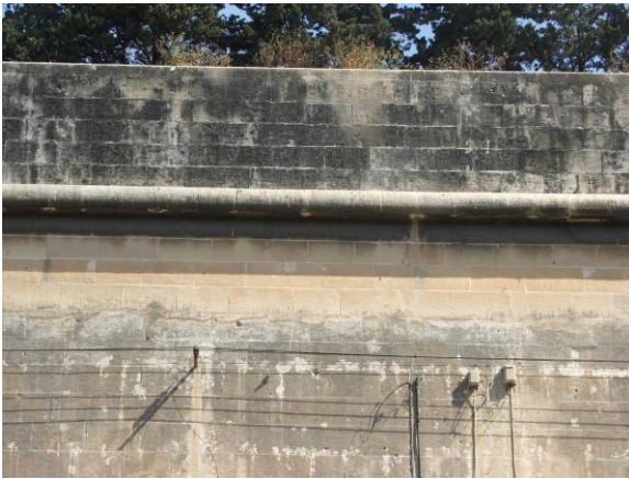
Fig. 13: Black crust and growth on parapet and cordon and accretions on scarp.
