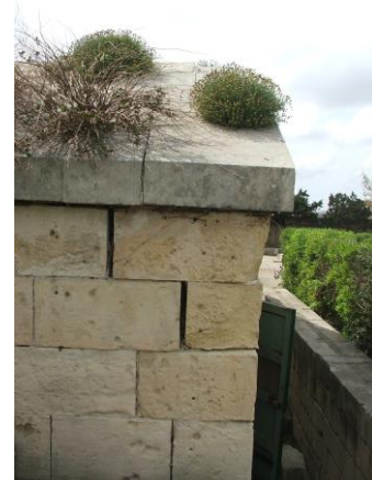
Fig. 37: Close-up of damage.
