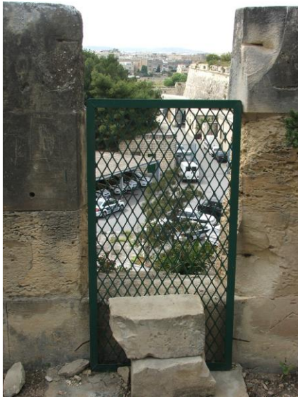
Fig. 24: Broken stone due to rust expansion and early alveolar decay.
