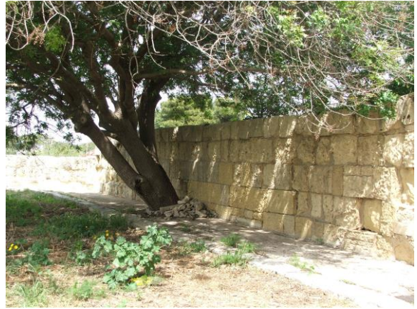
Trees in a sensitive corner and cement pointing.
