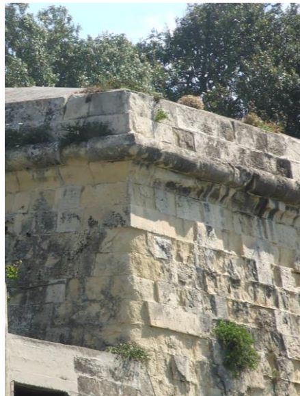
Broken quoins, erosion and crust on salient.
