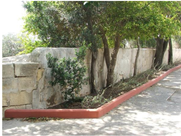
Missing banquette and trees planted in a sensitive location. Parapet is heavily plastered.
