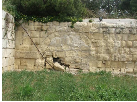
Badly deteriorated wall and blocked doorway.
