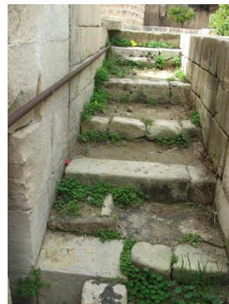
Fig. 39: Breakage due to accretions.
