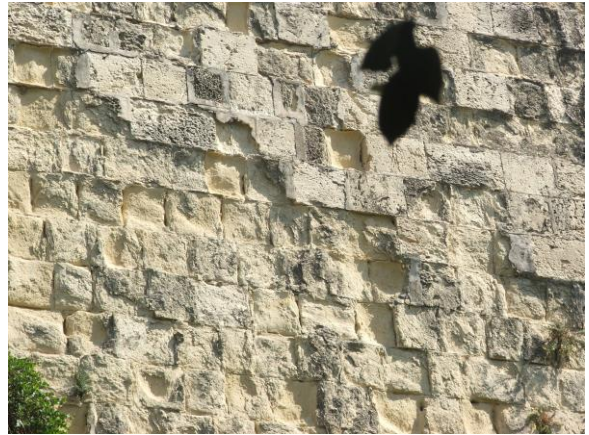
Only few areas of the masonry's patina remain.
