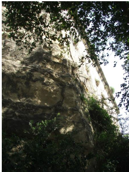
Tree hidden base of shoulder.
