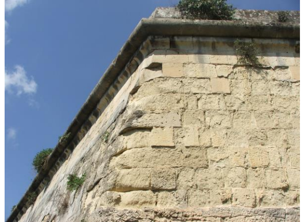
Badly broken and eroded quoins on shoulder.
