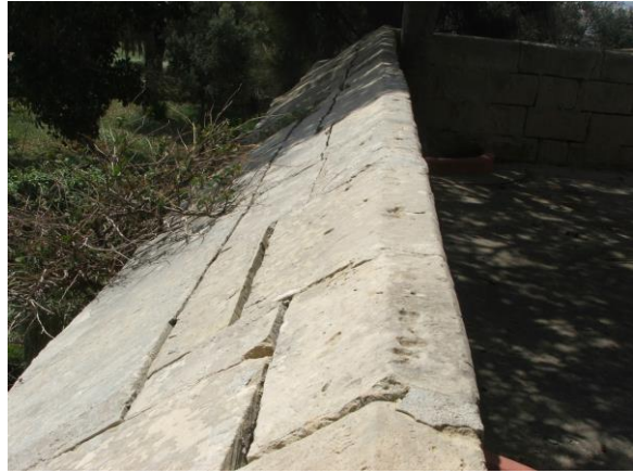
Dislodged quoins and voided mortar joints.
