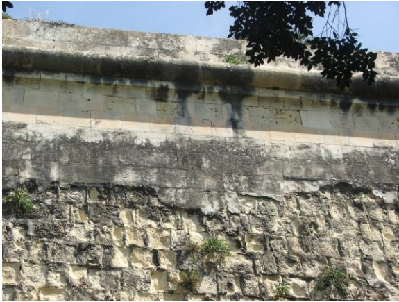
Delamination, black crust, powdering and growth.
