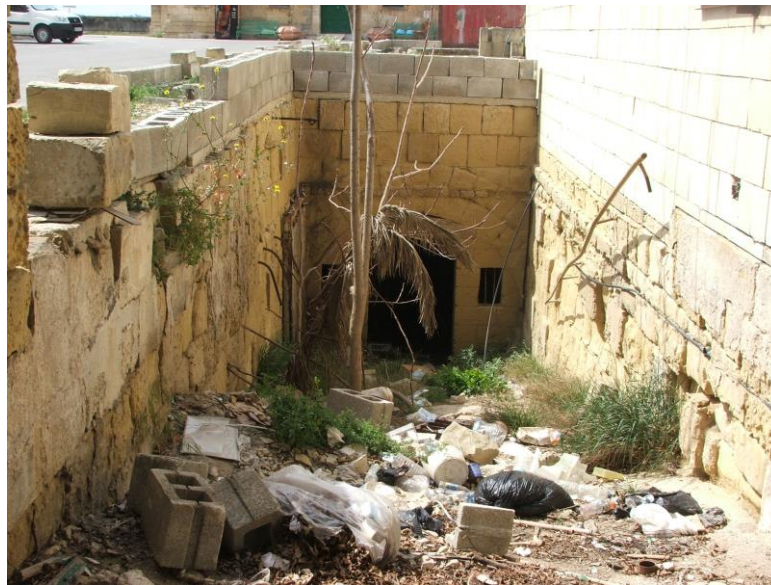
The badly deteriorated and rubbish infested entrance.
