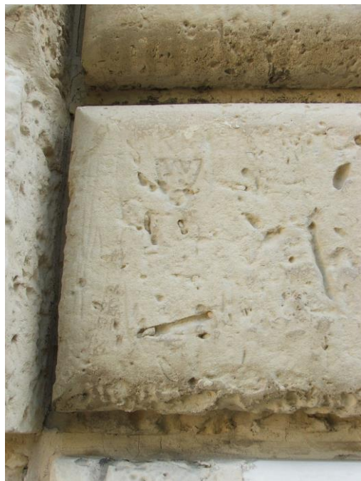
Deterioration and graffiti on masonry.
