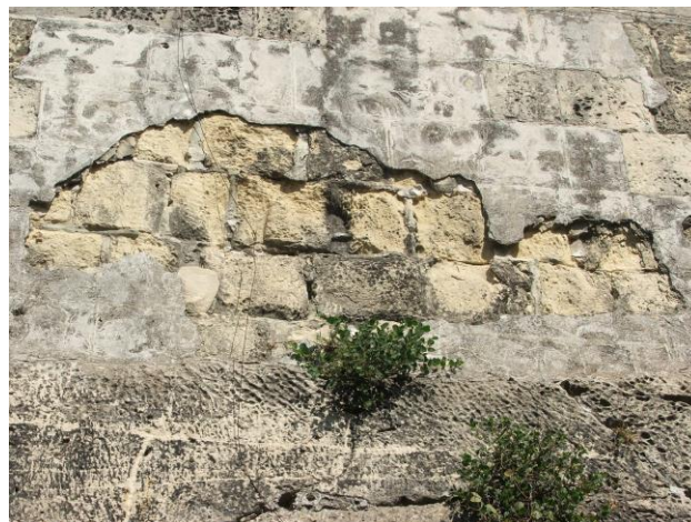
Fig. 47: Old plaster on deteriorated masonry.
