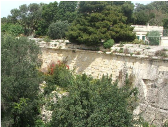
The deteriorated masonry face of the curtain.
