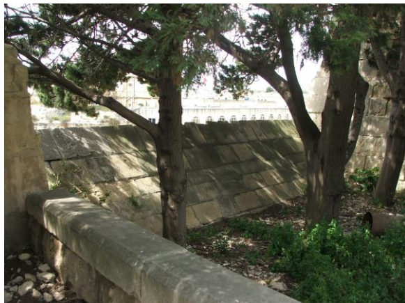
Fig. 29: Trees growing in gorge by batardeau. Heavy powdering and voided mortar joints.
