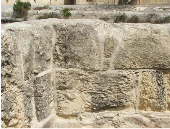
Cement pointing on corner of left shoulder.
