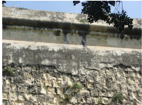
Fig. 44: Alveolar and other erosion, black crust and algae along face, cordon and parapet.
