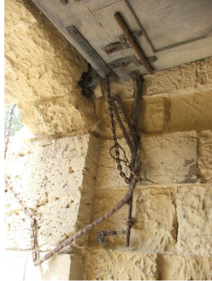
Eroded masonry and rusting fittings.
