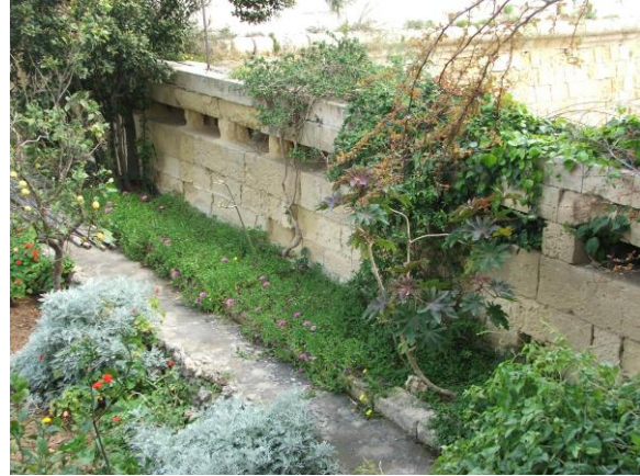
Eroded and infested musketry loop-holes.
