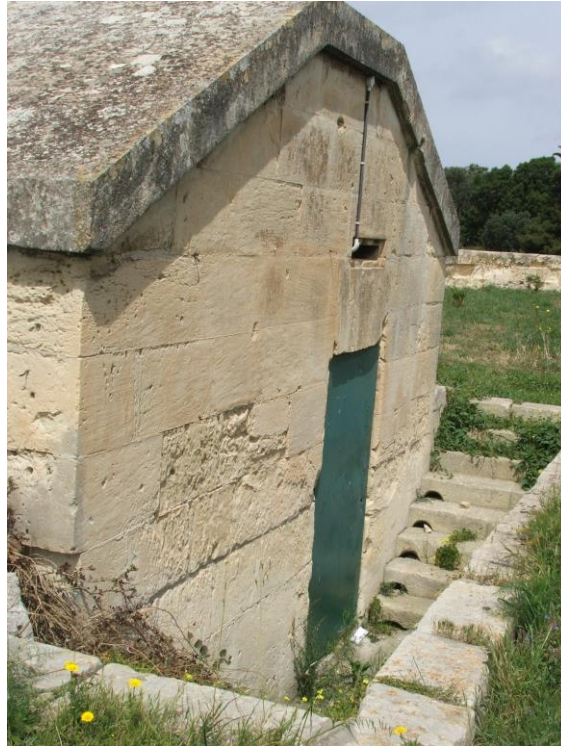
Identical deterioration on the right magazine.
