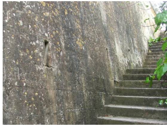
Fig. 41: Lichen, algae and fungi on left stairs and counterscarp.
