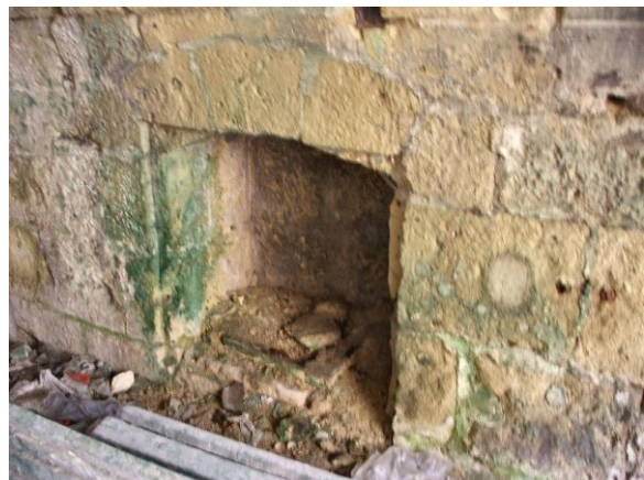
Moss and deterioration on the masonry fabric.
