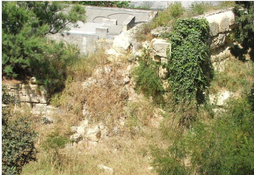
Badly damaged side of parapet by demi-bastion overgrown with plants and trees.
