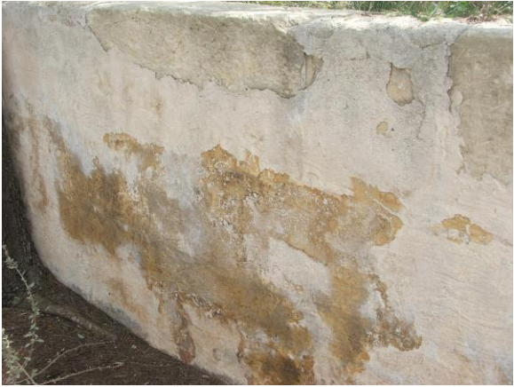
Parapet with heavy plastering and algae growth.
