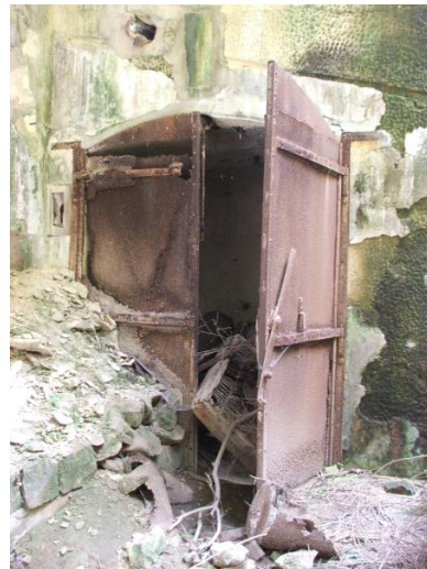
Moss encrusted walls, neglect and debris.
