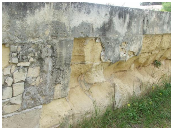
Erosion, cladding and rendering inside parapet.
