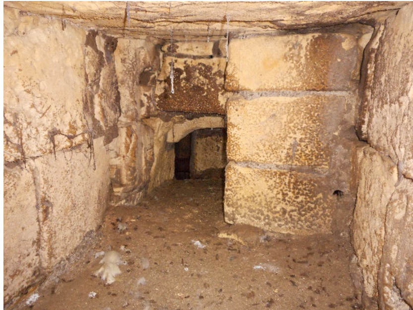
Fig. 63. Old sewer gallery under Marsamxett Street that once discharged into the sea.
