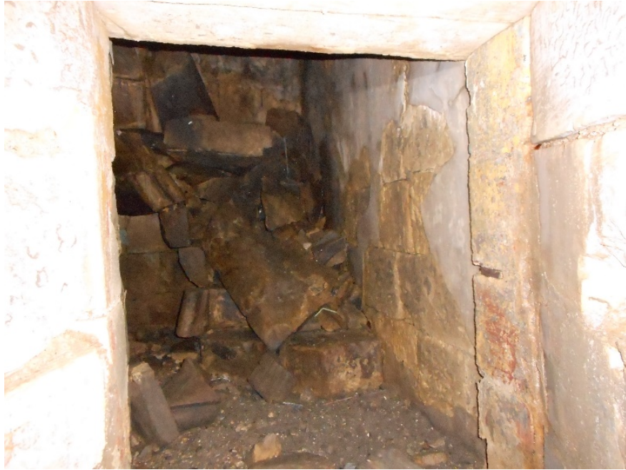
Fig. 61. Collapsed spiral staircase and doorway under Mattia Preti Square.
