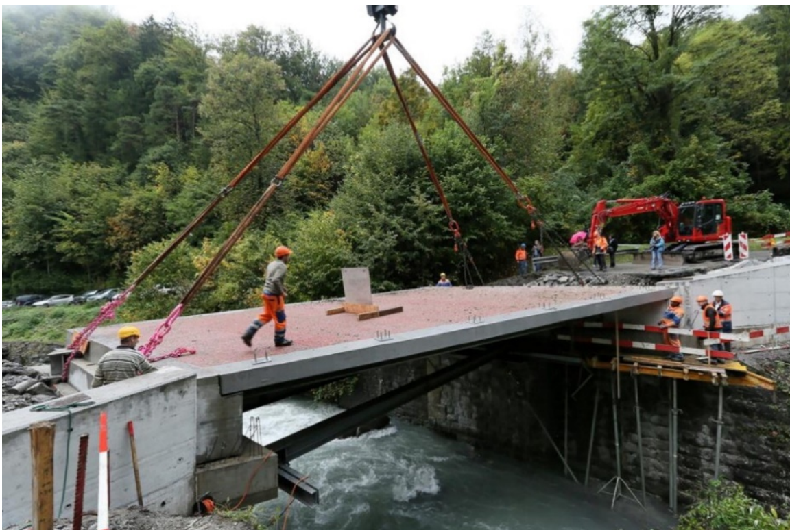
Figure 2-8: Vehicular bridge, Avancon River, Switzerland. Deck is composed of GFRP sandwich panels (Osei-Antwi, de Castro, Vassilopoulos, & Keller, 2013).
