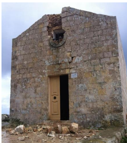
Figure 49 - Chapel of St Mary Magdalene Incident Struck by Lightning 2014 (Vassallo, 2014).
