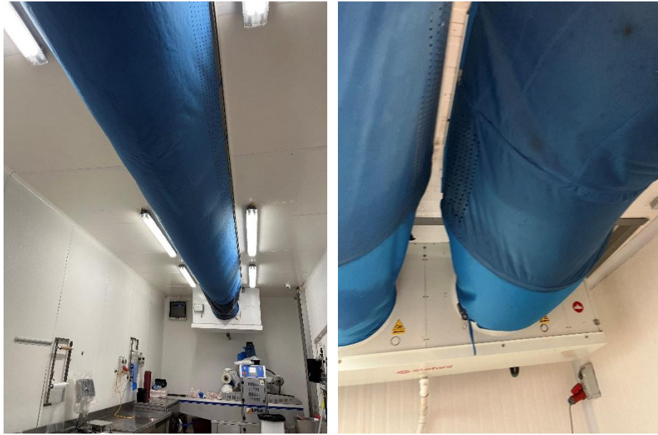
Figure 1.6 - Overhead cooling devices throughout the plant.
