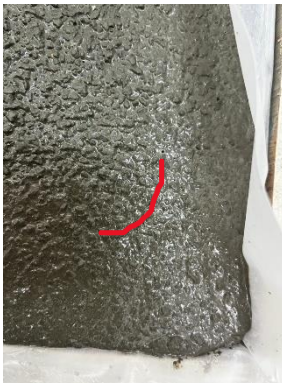
M0 – Crack Formation
