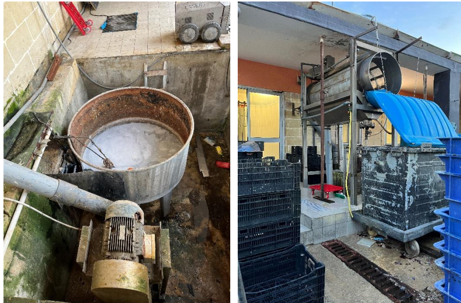
Figure 3.6 - (right) Collected waste is pumped up to the drum and (left) Drum which empties solids into the large plastic bin.
