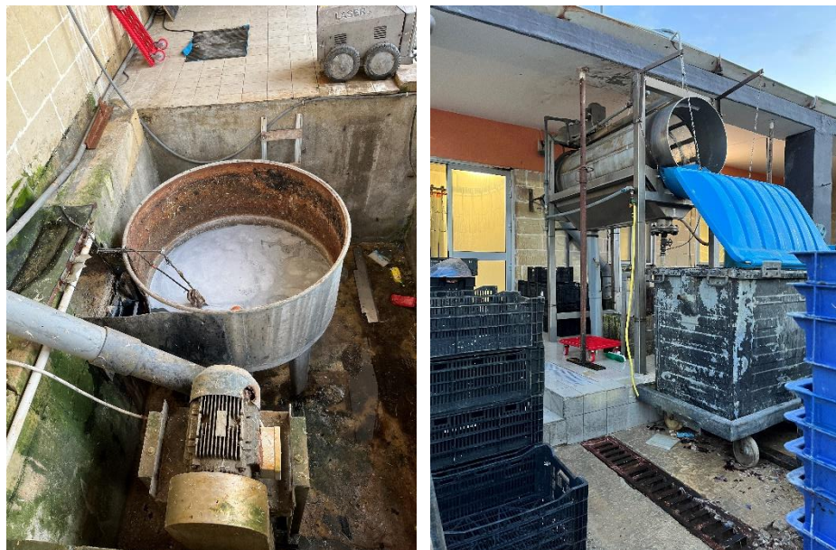
Figure 11 - (right) Collected waste is pumped up to the drum (left) Drum which empties solids into the large plastic bin.
