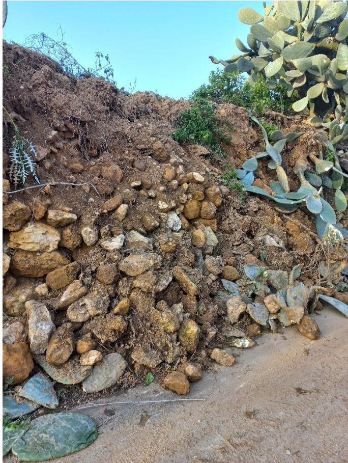
Figure A4-4: Another Effect of the Storm: Broken Rubble Walls
