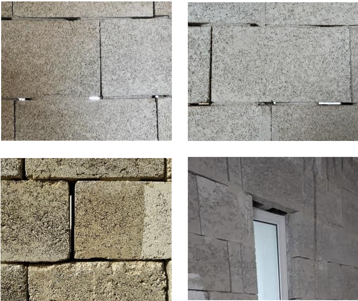
Figure 1.1: Examples of poor workmanship, Marsaskala, Malta
