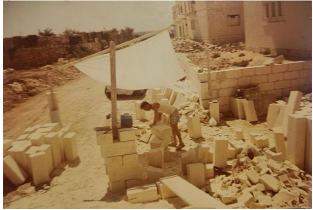
Fig. 2 A father (builder by profession) constructing a new home for his daughter and her fiancé on a state-provided Homeownership Scheme (HOS) plot, Haż-Żabbar, 1985. Source: Private collection
