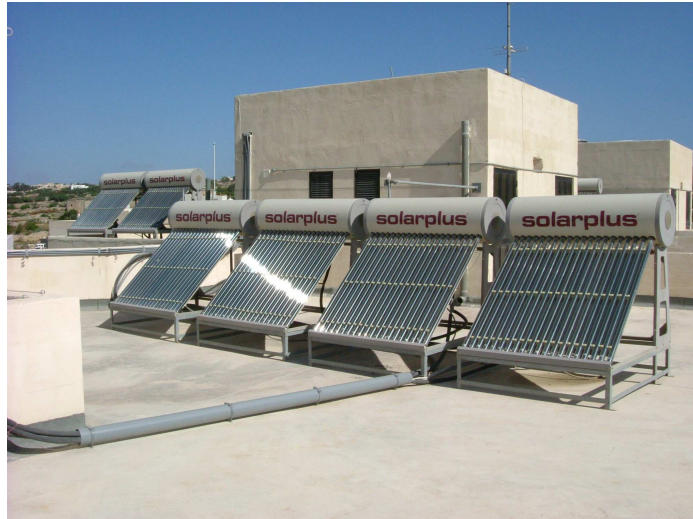
Figure 2: Solar water heating systems installed on the roof of the Sustainable Housing Project at Tal-Ftieh, Birkirkara, Malta.
