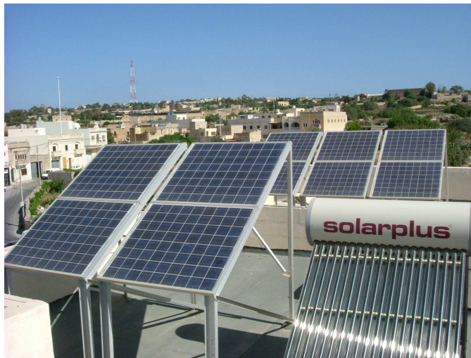
Figure 3: The 1.5 kWp Photovoltaic system, comprising 10no. modules and an inverter, connected to the showroom of the Housing Project.
