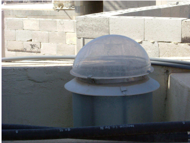
Figure 4: One typical sun pipe installed and capped at roof level, running down through the shaft to the underlying garages at basement level.
