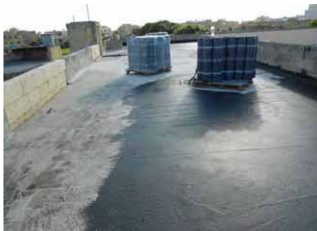
Works during the reinstatement of the main roof of the Gozo Campus.
