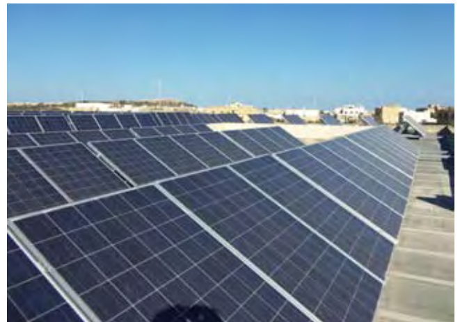
Photovoltaic panels on the roof of the Gozo Campus.
