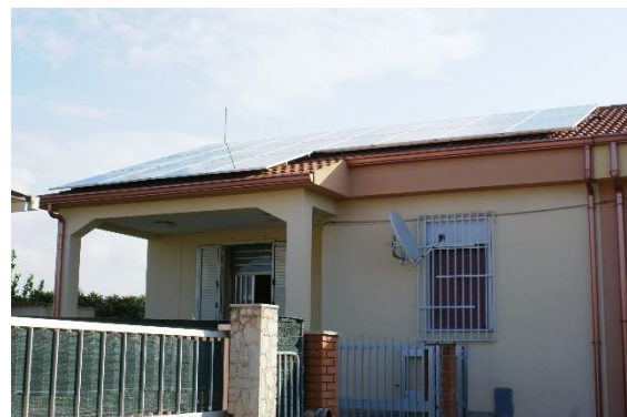
Figure 3: PV system in a dwelling (Santa Croce)
