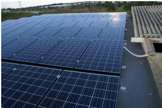
Figure 2: 30 kWp PV system in Pozzallo.
