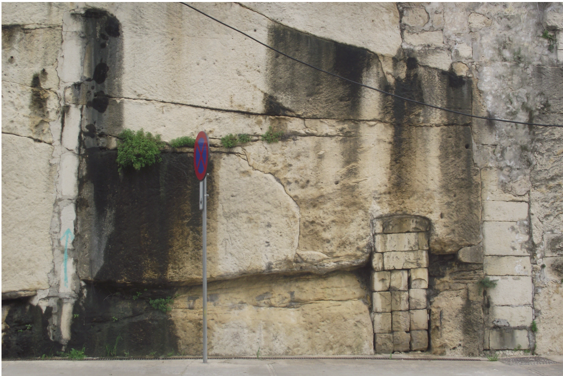
Fig. 2 Example of ground water flowing along a bedding plane, exposed by a modern cutting along the Marsa-Floriana shoreline
