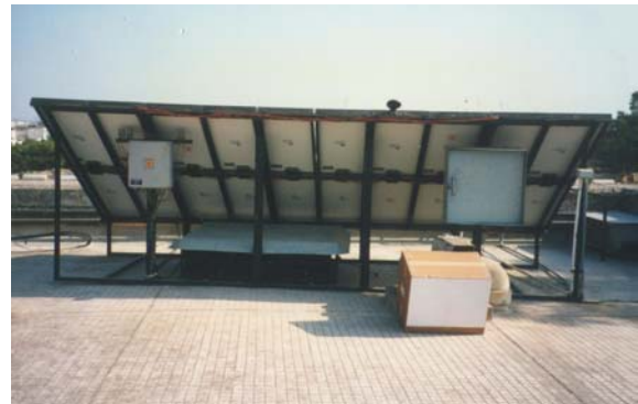
Figure 2: The first solar PV stand-alone system to be tested in Malta (1993-1995). A battery bank was placed underneath the modules and a battery charge control unit is seen to the left. Monitoring equipment was placed in the box to the right.
