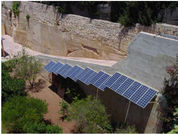
Figure 5: The first 1.5 kWp privately owned residential solar photovoltaic grid-connected system installed in May 2002, Madliena, Malta.
