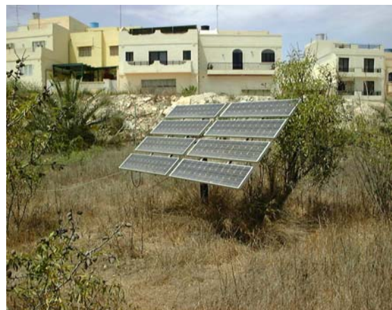
Figure 1: A solar photovoltaic water pumping system, installed at the Institute for Energy Technology since 1985.
