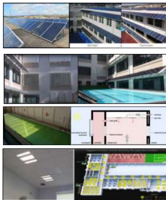
Figure 2: From top left to bottom right : Roof mounted photovoltaics, wall mounted photovoltaics also acting as overhangs, BMS controlled, automated lovers, pool solar water heating, automated pool cover, CO 2 controlled mechanical ventilation system, Intelligent lighting using photocells + soffit mounted infra-red panel heaters and the fully fledged BMS
