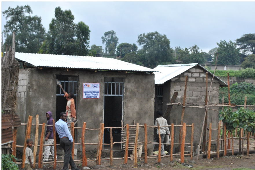
Left: Workers finishing off the construction of the biogas generator in the city of Shashamene
