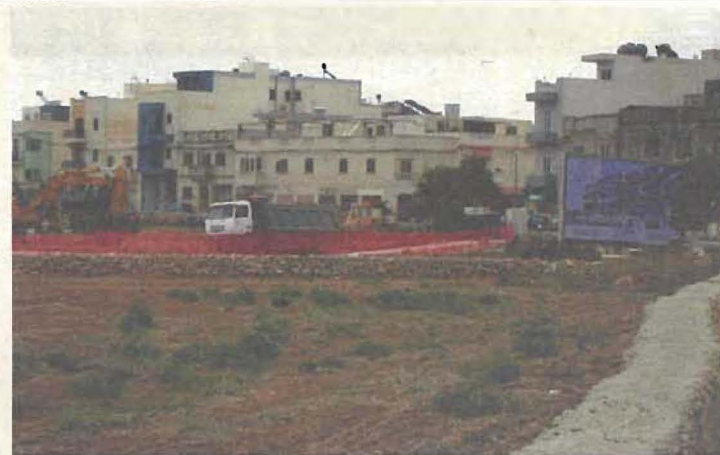
When revising local plans and development boundaries, the mistakes made in 2006 should be avoided. Seen above are maisonettes developed in a former ODZ site in Attard.
