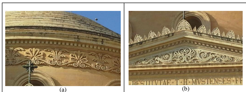
Figure 3. Details from Figure 2b: (a) cornice with lotus and honeysuckle ornament in relief and (b) pediment, the ornament in relief was introduced after 1860.
