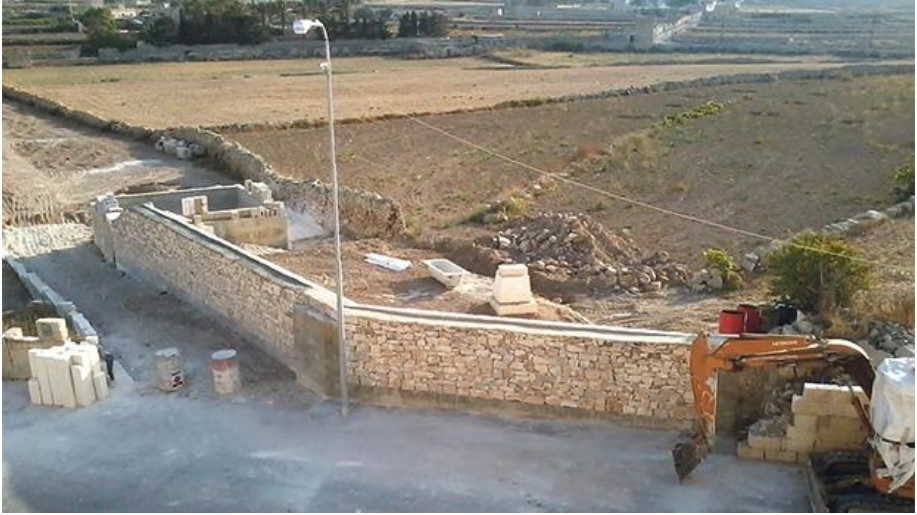
Sequence of works on a site in Siggiewi. The applicant has been granted a permit for an ODZ terrace with a view in the middle of fields, on the back of a number of dubious pretences. Architect: Robert Musumeci.
