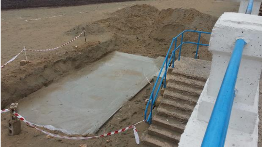
Laying the concrete foundations for yet another kiosk at Ghadira, without due environmental assessments having been done on a beach where public space is already at a premium. Photo: Caroline Muscat
