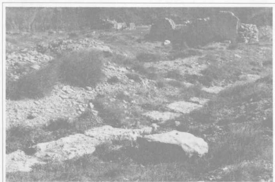
Plate 1a. RAS IR-RAHEB: Detail of remains showing line of foundation walls and the two megalithic blocks in February 1988.
