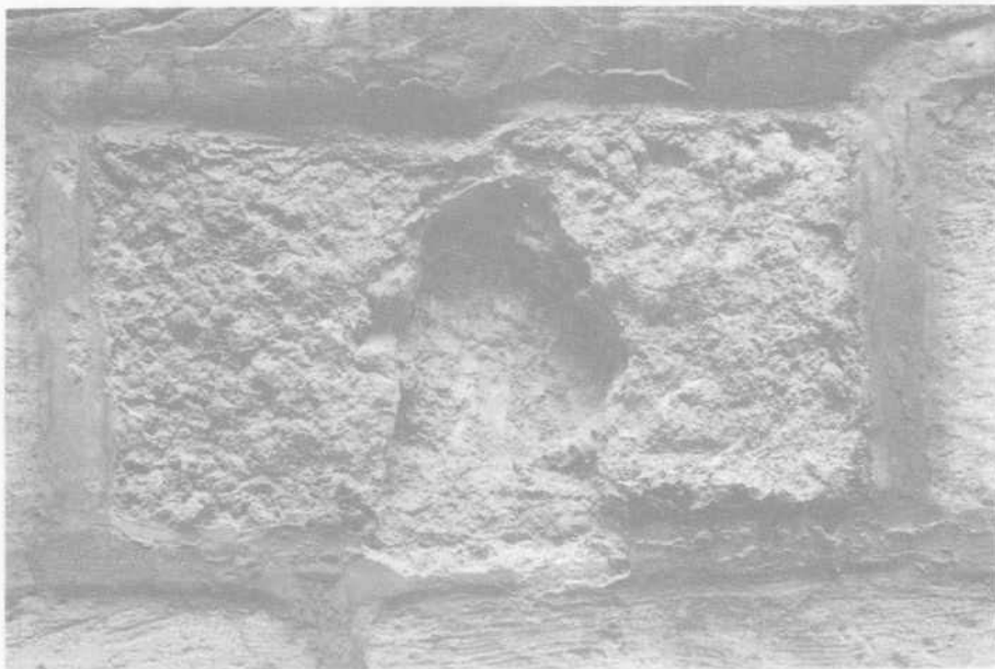
Fig. 2: Badly-deteriorated block of stone in the inner yard of the Upper Prisons (block 1 in Fig. 4). This block now has no graffiti, though it may have originally had one.
