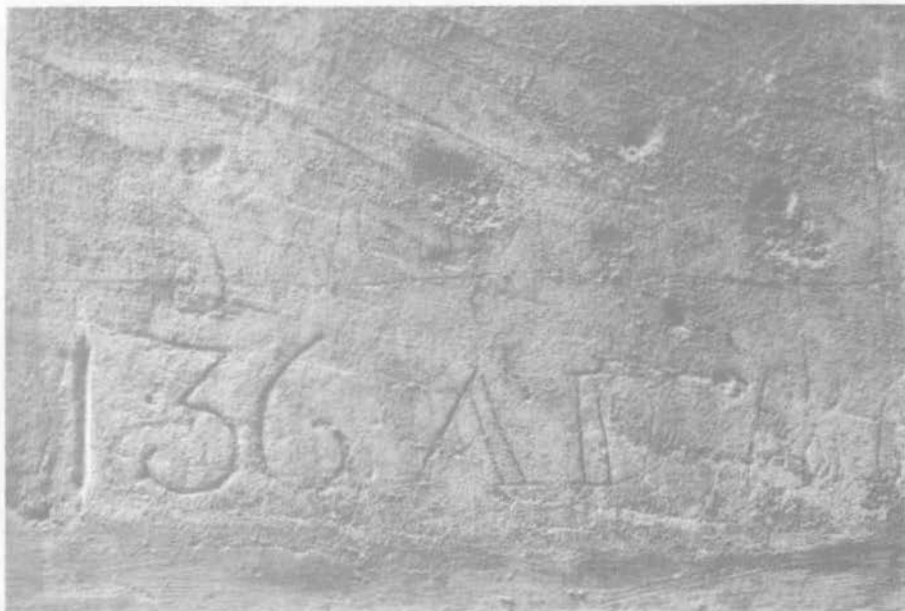
Fig. 5: One of the graffiti in the corridor of the Upper Prisons, in a good state of conservation. Note, however, the presence of mould, and the incipient deterioration of the stone surface.
