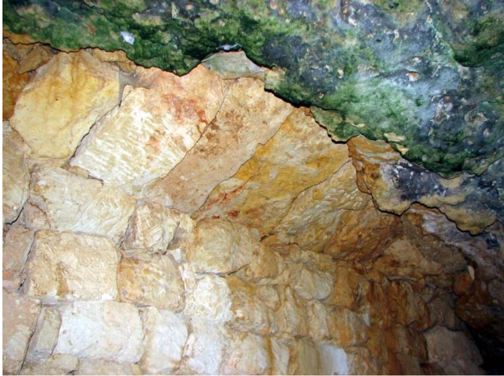
Plate 16 Roughly faced ashlars bridging the gap between the cave-roof and the dry-stone screening wall.
