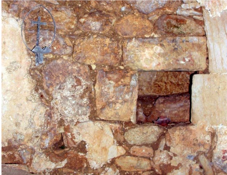
Plate 6 Detail of wall-niche in the southeast corner of the apse, probably used for the keeping of sacred vessels.
