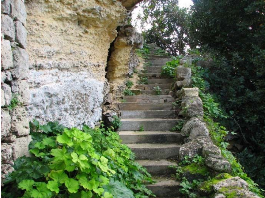
Plate 3 Concrete-clad footpath and steps giving access to the cave-church entrance. Fissures in the rock-face are symptomatic of cliff-face detachment.
