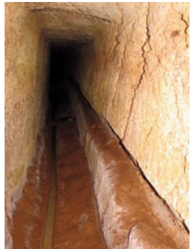
Fig. 10.8. Canals are often carved into the floors of galleries in order to ease the water flow retrieved from the perched aquifer.
