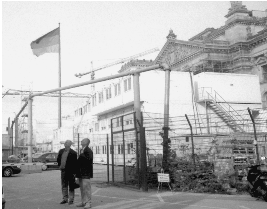
A behind the scenes view of the reconstruction of the Reichstag in 1998. This figure was taken only months before the German Parliament was to again take its seat in Berlin. Yet the Reichstag is a symbol of mixed meanings, the house where the will of the German people was exercised, as well as the place where German democracy was curtailed and overthrown.
