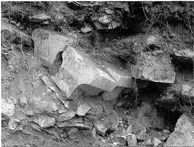
Plate 5. Roof collapse behind the main altar
