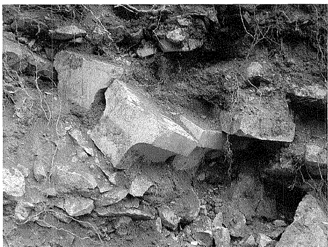
Plate 5. Roof collapse behind the main altar
