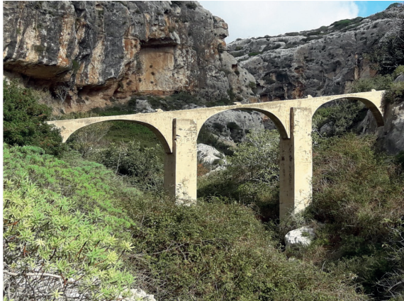
Figure 4b. The three arched concrete bridge intended to support the water pipeline, crossing the valley.
