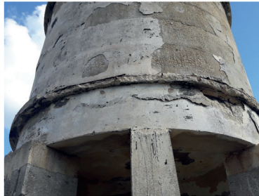
Figure 3c. Degradation in the water tank and ring beam including cracking and spalling as a result of the corrosion of the reinforcement.
