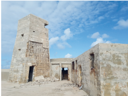
Figure 5a. The Bastion No.4, twin 6-pdr QF gun emplacement with the characteristic high fire control tower at Fort Ricasoli.
