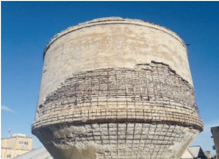
Figure 2a. Degradation on the south face of the tank, corrosion of reinforcement, spalling and delamination of concrete.
