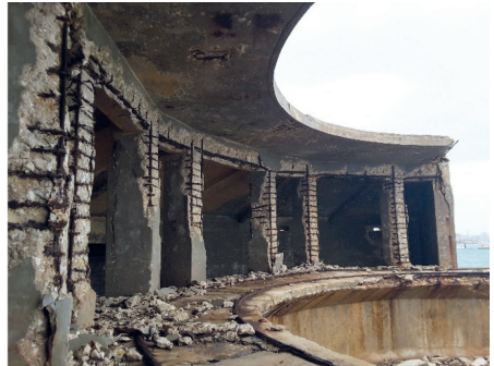
Figure 5b. The passageway and overhead protection at the back of the twin 6-pdr QF gun emplacement at Fort Ricasoli, with severe degradation.
