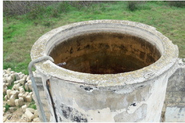
Figure 3b. Water Tank.
