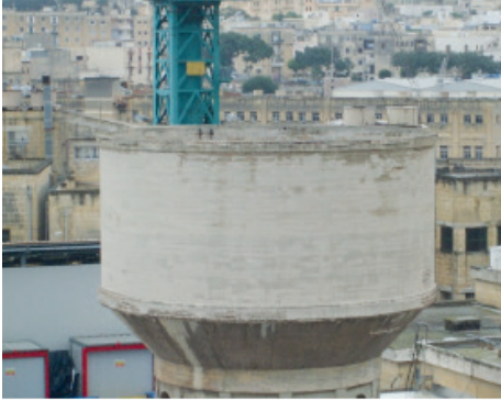
Figure 1b. The upper part of the structure consisting of a reinforced concrete tank.
