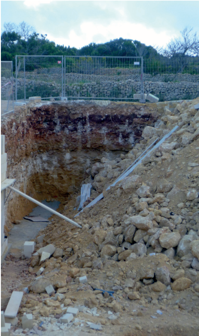
Figure 5.14 (above). A typical terra rossa soil sequence in Xaghra town at construction site 2 (C. French).
