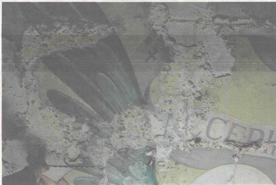
Deterioration of the nave marouflage paintings.
