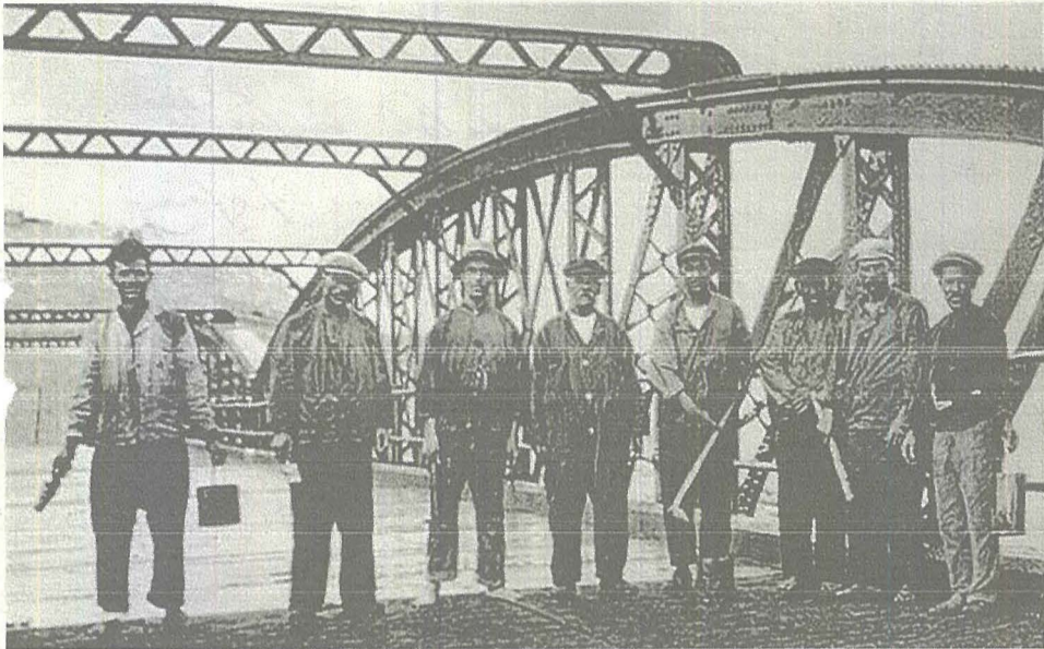
A gang of eight workmen painting the footbridge. A good number of the workmen were foreigners.
