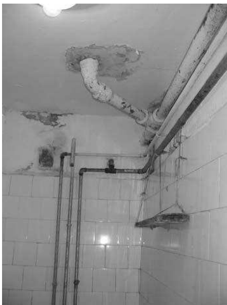
c. Degradation of the tiles and piping
