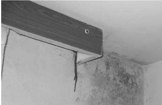
a. Mouldiness on the exterior walls
