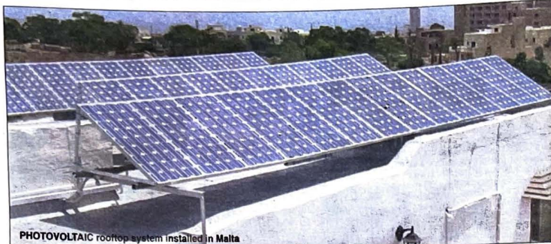
PHOTOVOLTAIC rooftop system installed in Malta
