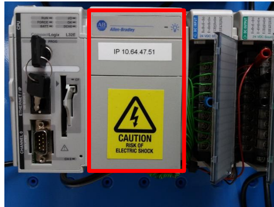
Figure 8: PLC power panel
